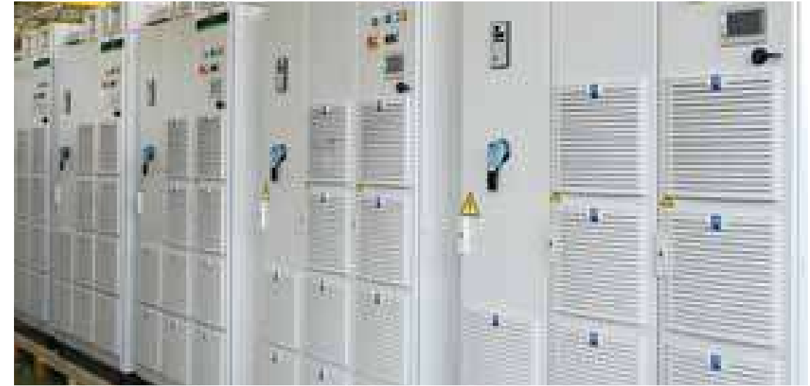
Variable speed drives panels
